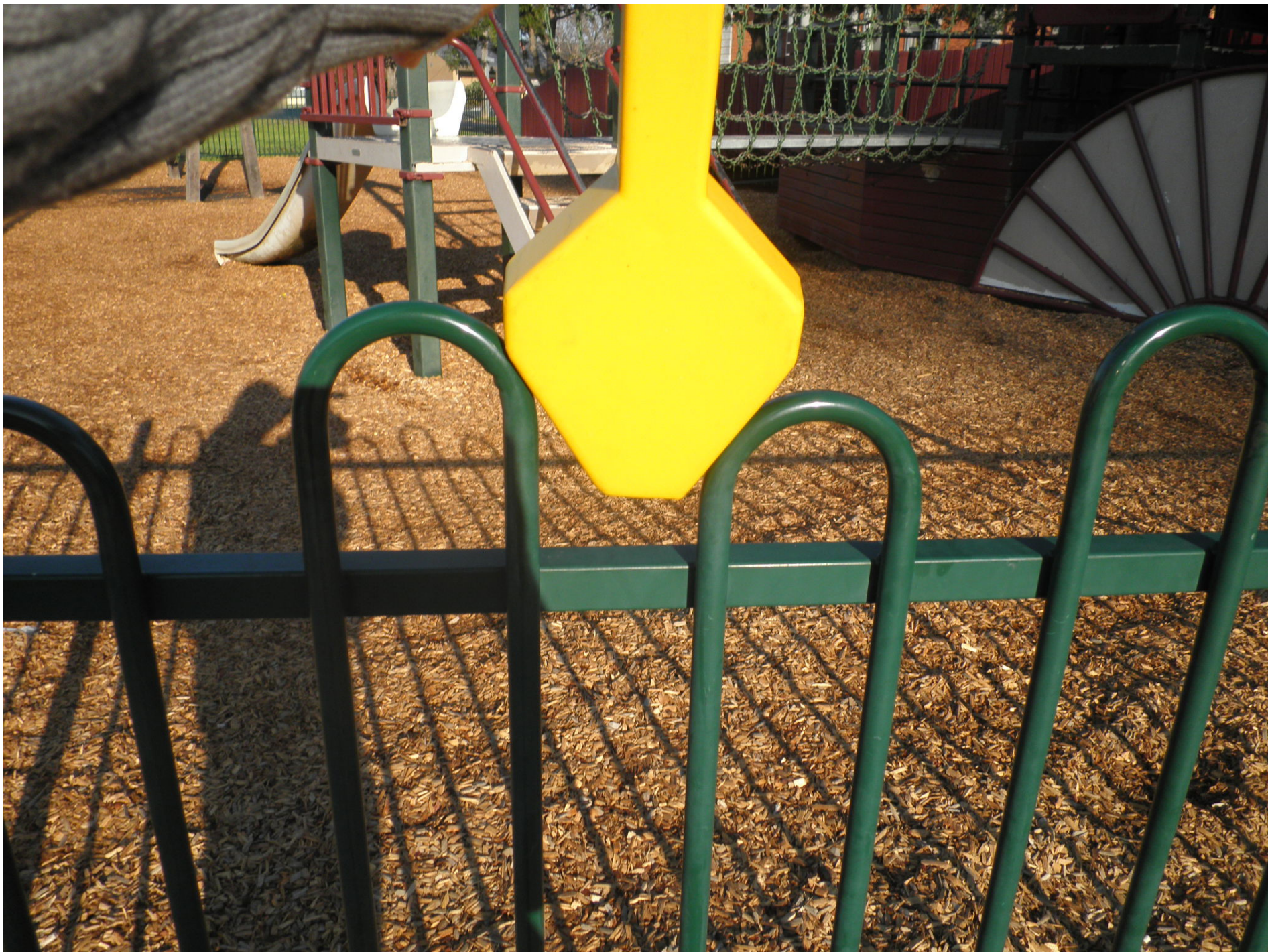
Potential neck traps top of fence – not play equipment but not recommended!
